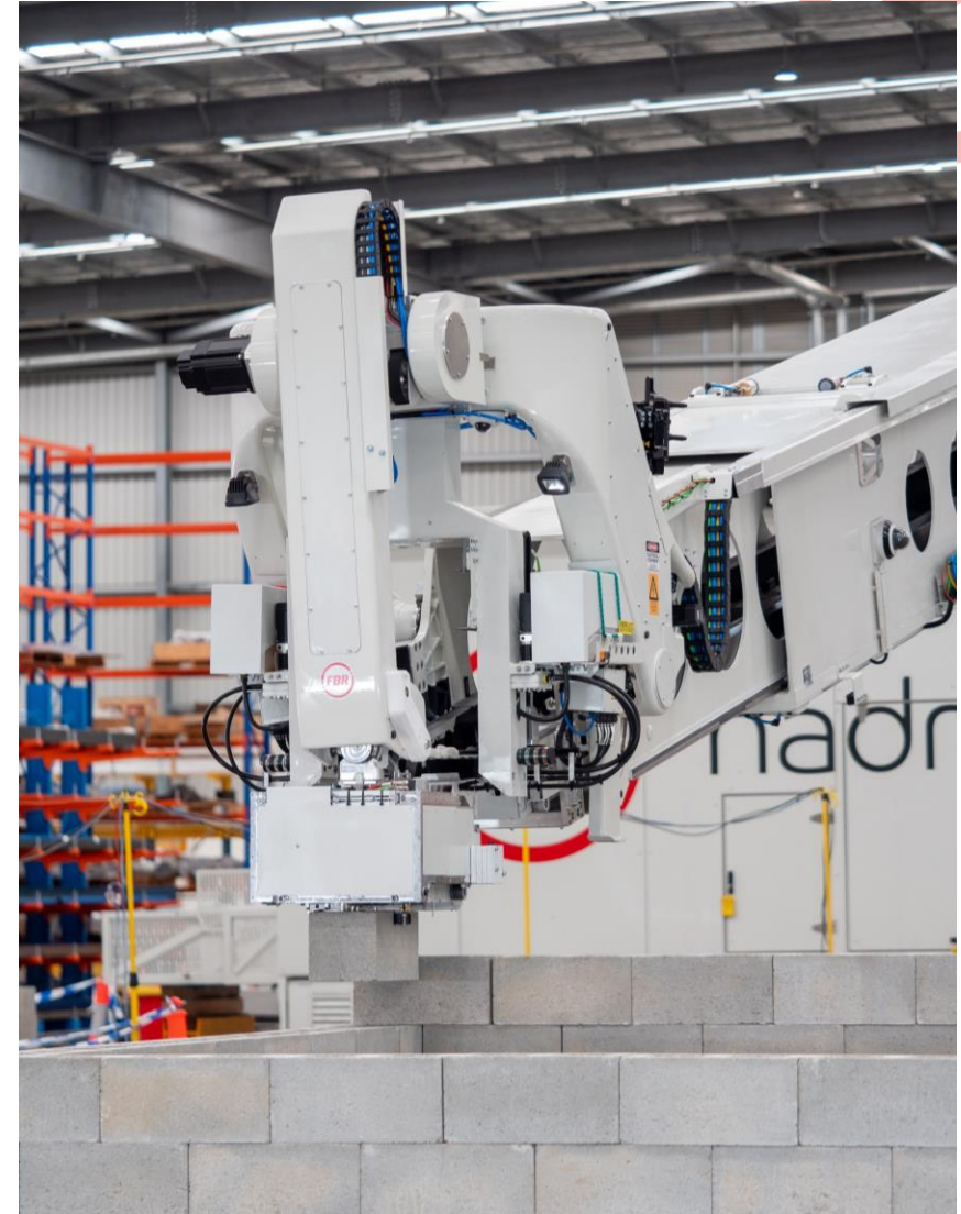
Next-generation Hadrian X ® builds test structure with lay-path vectoring to close perpendicular gaps
