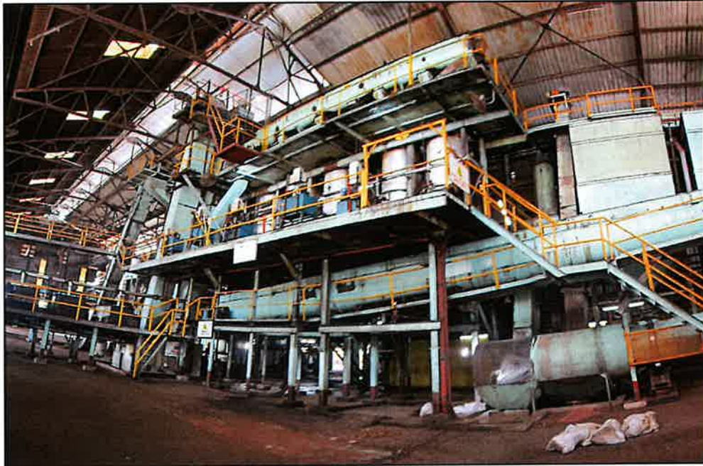
VIEW OF PRESS STATION
