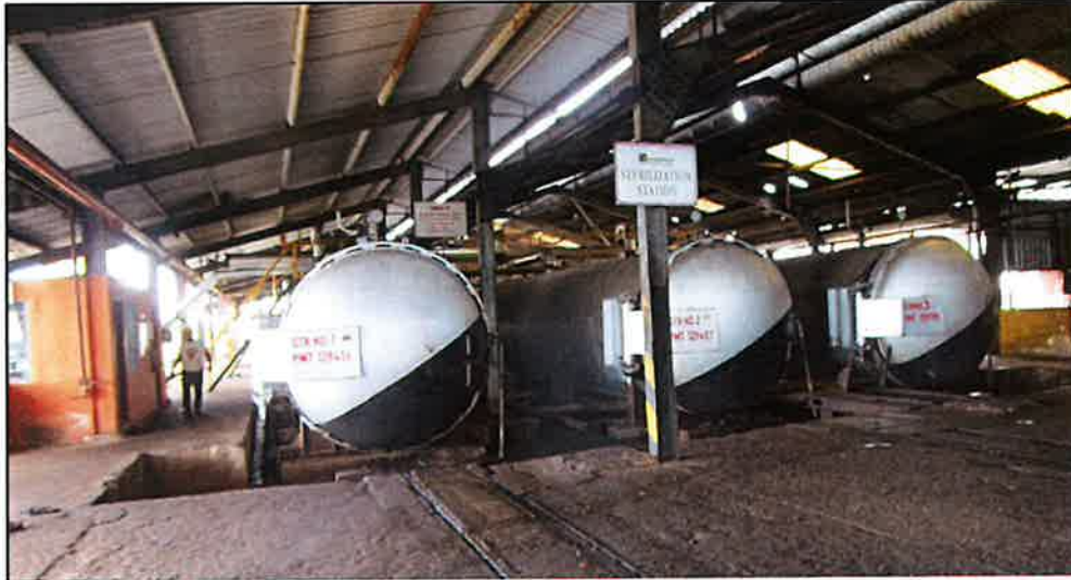
VIEW OF STERELISATION STATION
