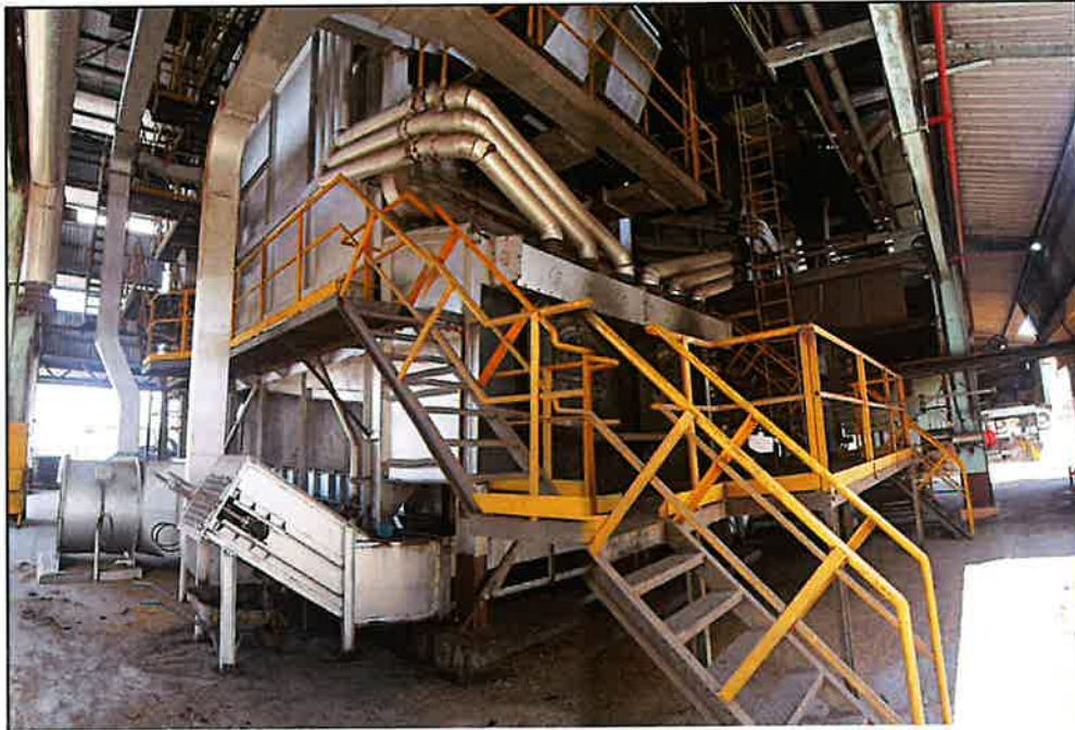
VIEW OF BOILER
