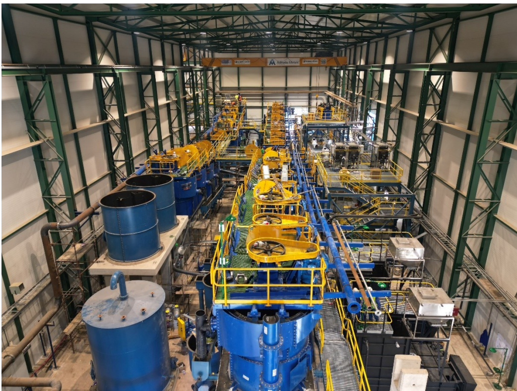
Figure 8: Looking south in zinc flotation circuit, September 2023
