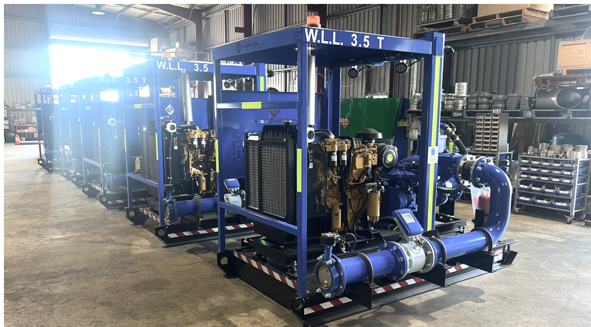
Figure 2: Industrial Diesel Pump Sets Supplied by PPS Undergoing Upgrades & Testing at PPS-Darwin
