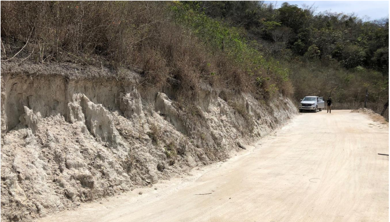
Figure 5: Highly weathered coarse quartz rich road cut at Carai which extends for 80m and sits below artisanal mine workings.
