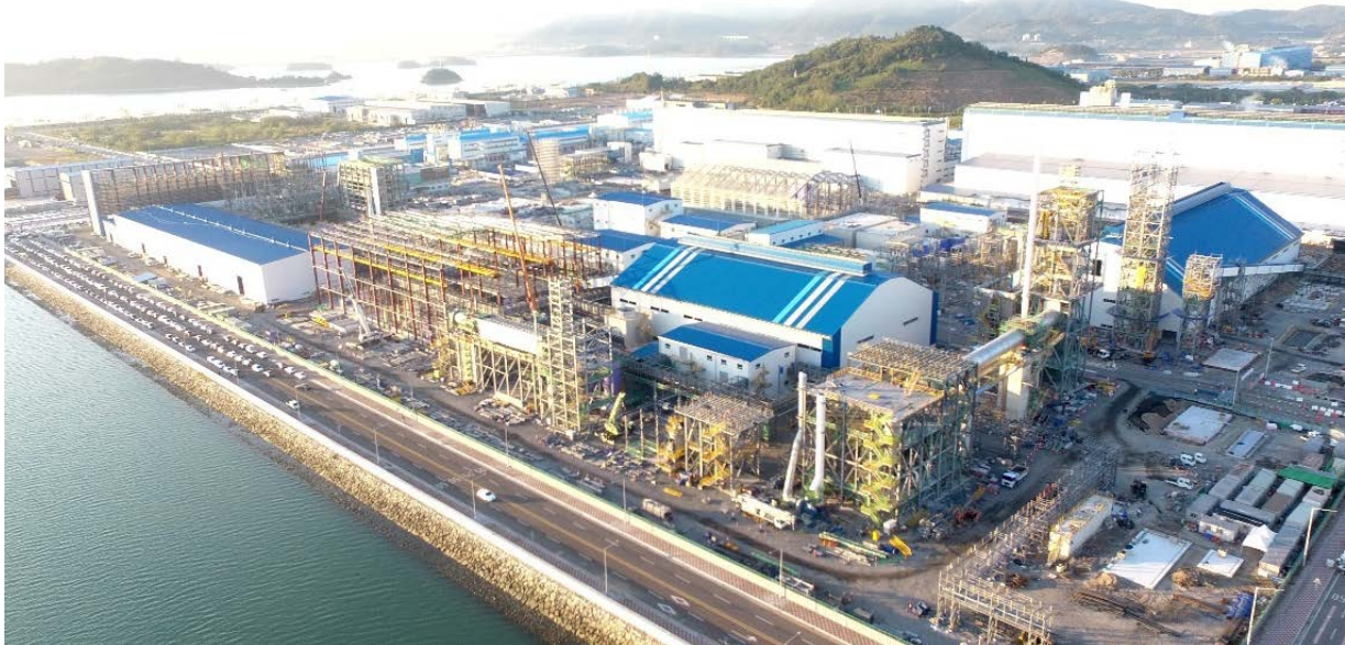
Figure 3: Construction site at the POSCO Pilbara Lithium Solutions LHM facility as at 18 October 2023
