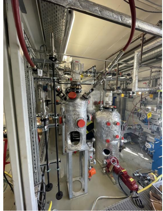
Figure 5 The Inlet Brine Cooling system
