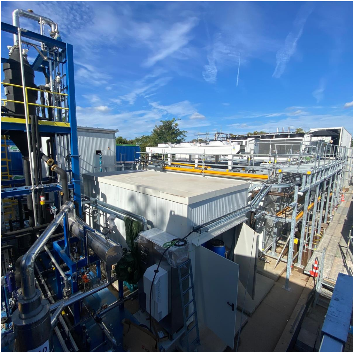
Figure 3 Overlooking Vulcan's Lithium Extraction Optimisation Plant.
