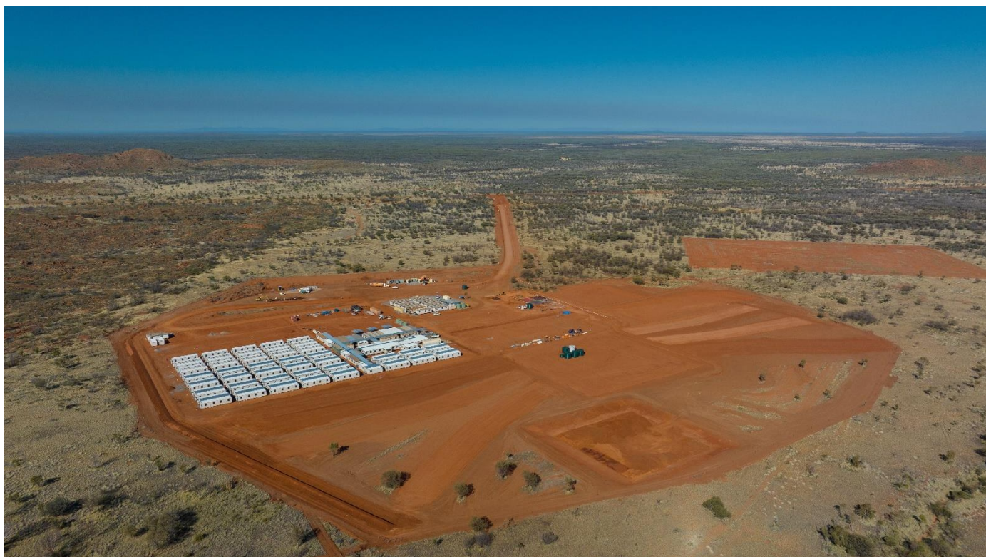
Figure 1: Aerial view of the Nolans Project village area, construction camp stages 1 and 2 at left, August 2023
