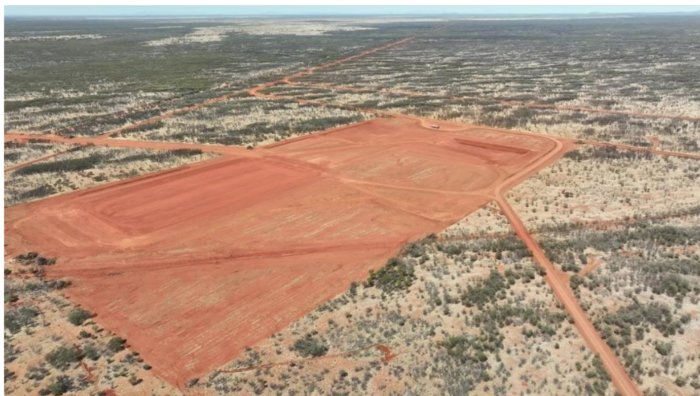
Figure 6: Process plant laydown area and concrete batch plant bulk earthworks complete, September 2023
