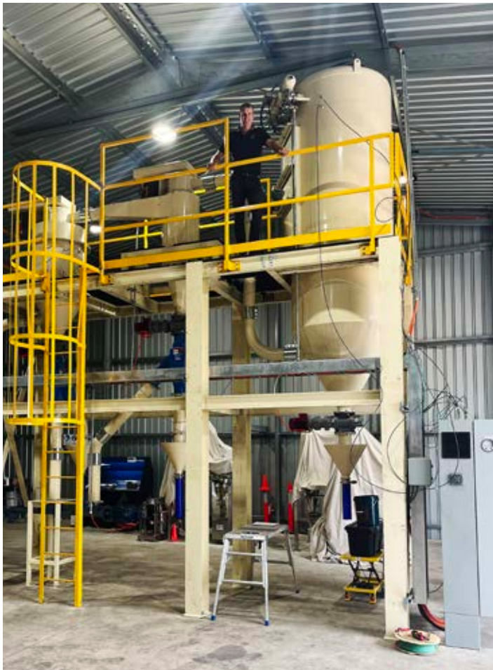
Figure 5: Qualification plant installation at International Graphite's R&D facility, in Collie, Western Australia.
