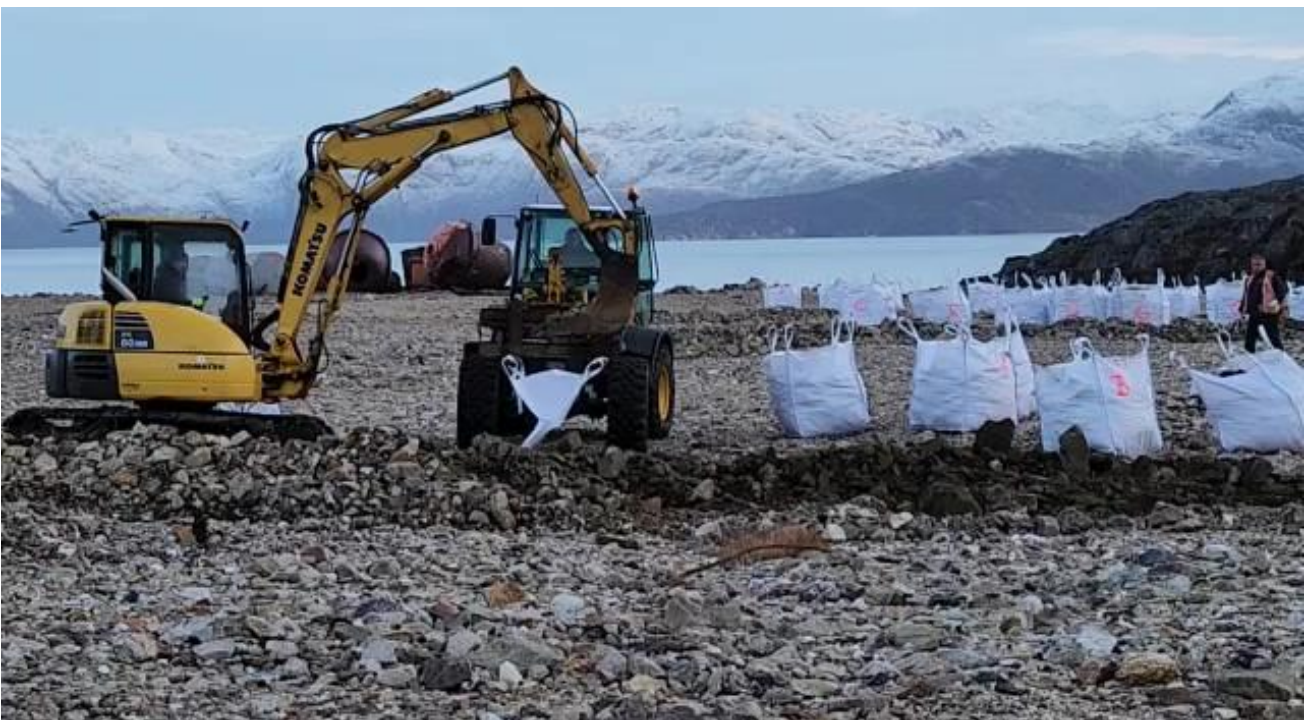
Figure 80: Collecting several tonnes of bulk samples from 5 trenches in the mineralized dumps
