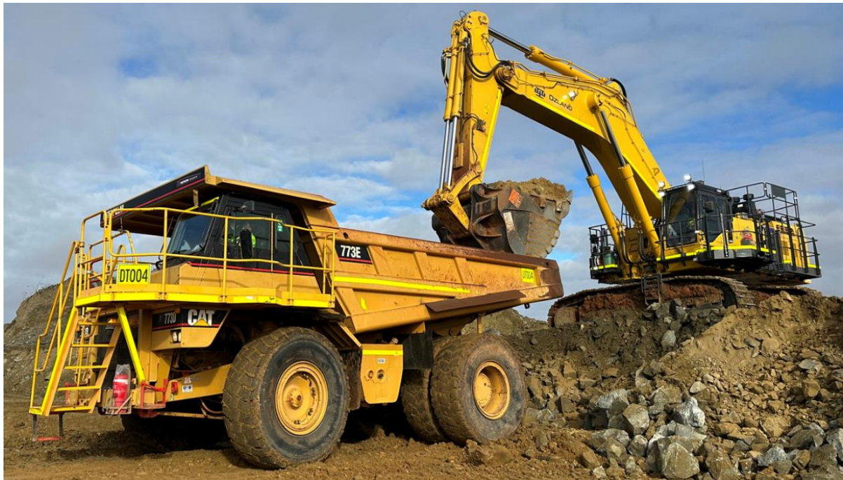
Figure 1: First load of waste from Greenfields loaded to complete TSF platform construction
