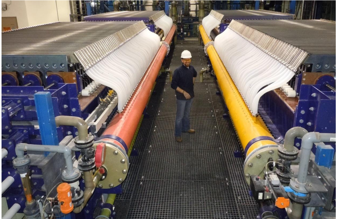
Figure 3: Two electrolyzers in an operational environment (Source: Ineos)
