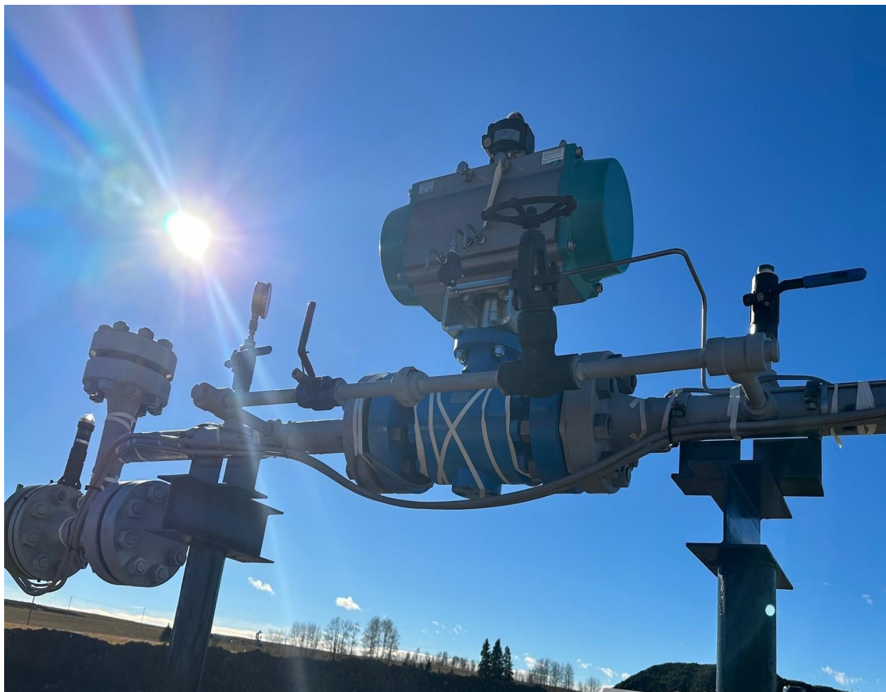
Figure 1. Certus 01-27-33-05 well flowline with gas metering device
