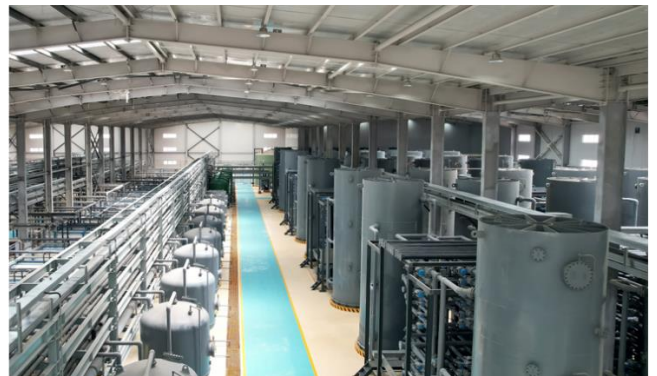
CHINA - EVEBATTERY 10,000 TPA LCE COMMERCIAL PLANT BUILT WITH SUNRESIN
