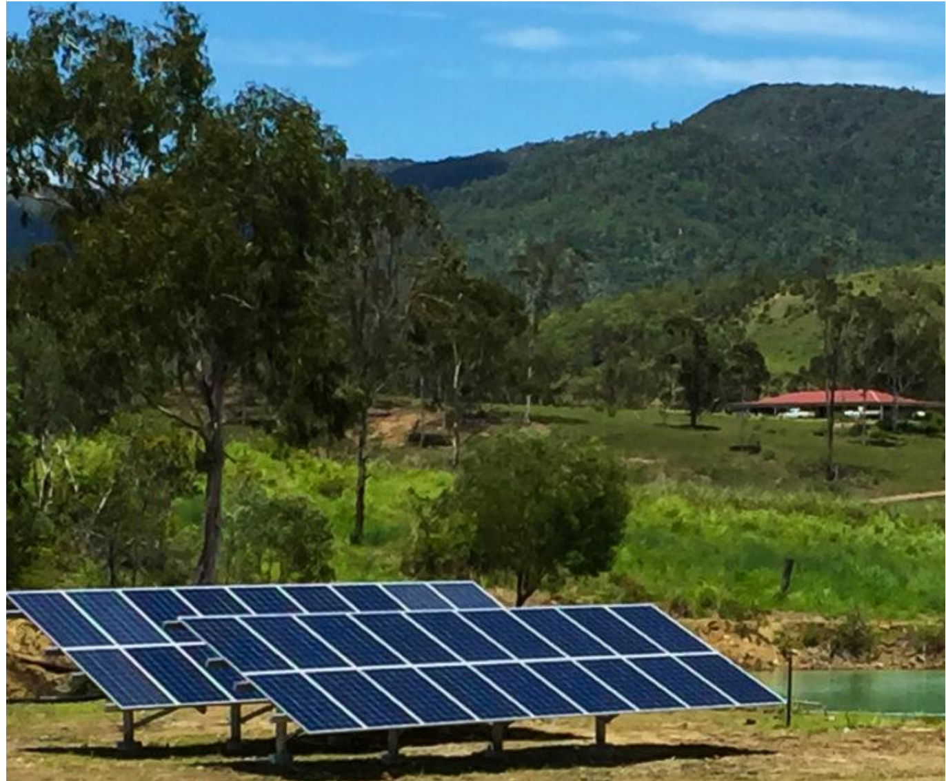
Solar Panels Onsite at the Mt Chalmers Mine.
