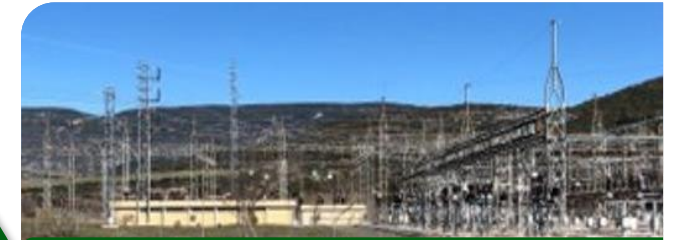
National Electricity Grid Substation in Sangüesa
