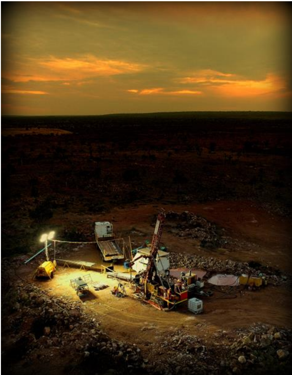
Figure 6: Browns Range HRE Project: Wolverine Deposit Resource Definition drilling program November 2023. HOLEID: BRWD0070.
