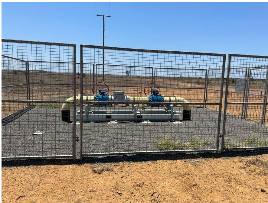
Figure: One of the QPME tie in points
