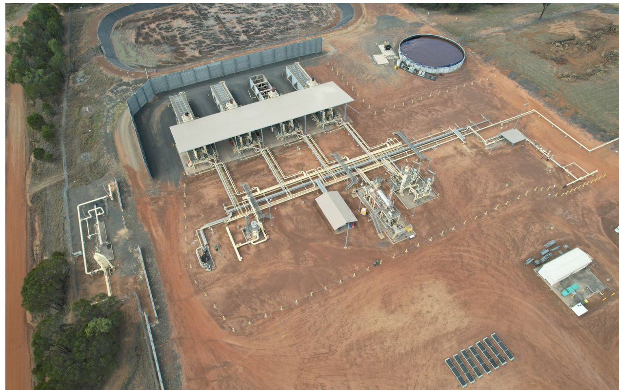
Moranbah Gas Processing Facility
