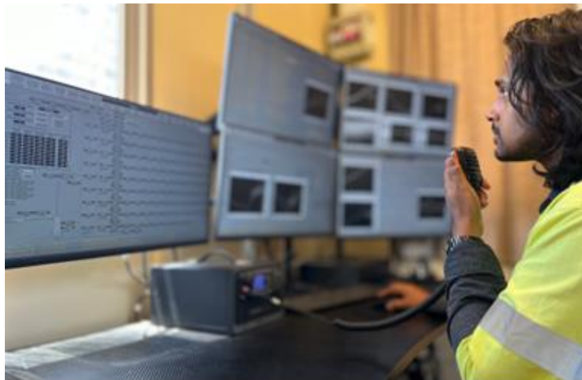
Control panel operator monitoring reactor heat up from the CDP control room
