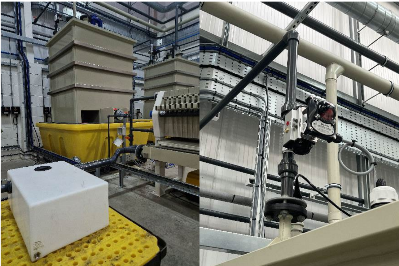
Figure 1: Reactor and Filter Press (shown in Figure 3 right) and automatic ball valve for feeding Reactor (right).
