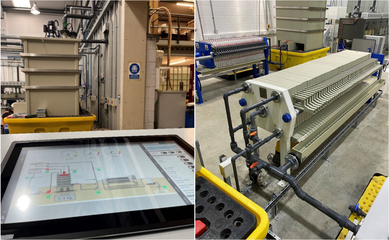
Figure 3: Left, Scada control panel in front of reactor vessel, and right, new digestion product filter.
