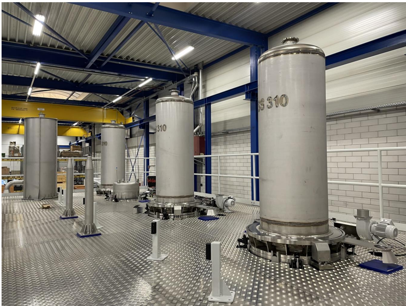
Figure 3: HAMR furnace retorts
