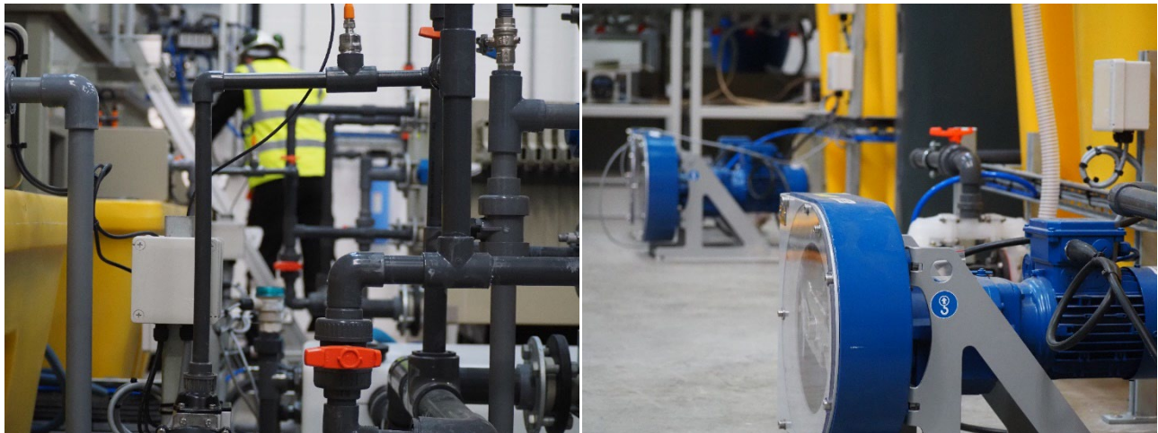
Figure 5: Left, Digestion outlet pipework and valves, and right, Separation circuit feed pumps.
