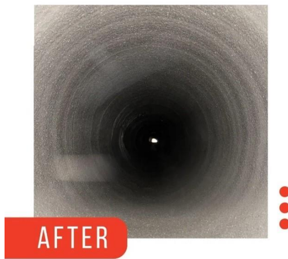
Figure 3. Worn pipeline after re-habilitation
