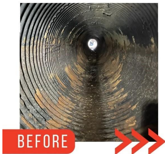
Figure 2. Worn pipeline before re-habilitation
