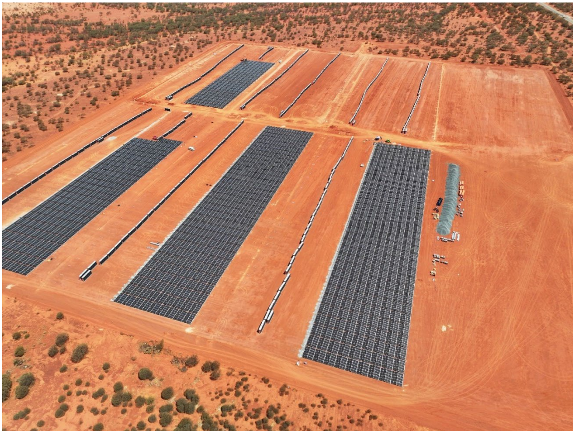
Figure 2: Installation of first 20MW of renewable energy solar power as at 21 January 2024.
