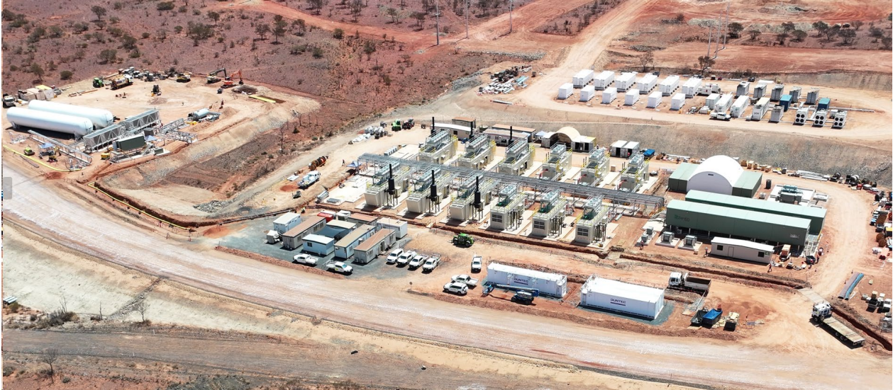
Figure 3: Thermal power station installation as at 21 January 2024 (including battery installation to the top of image).
