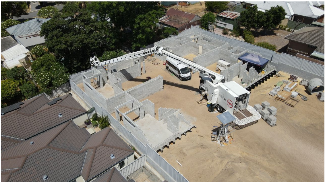
H02 constructing the walls of the first two townhouses at the St James site
