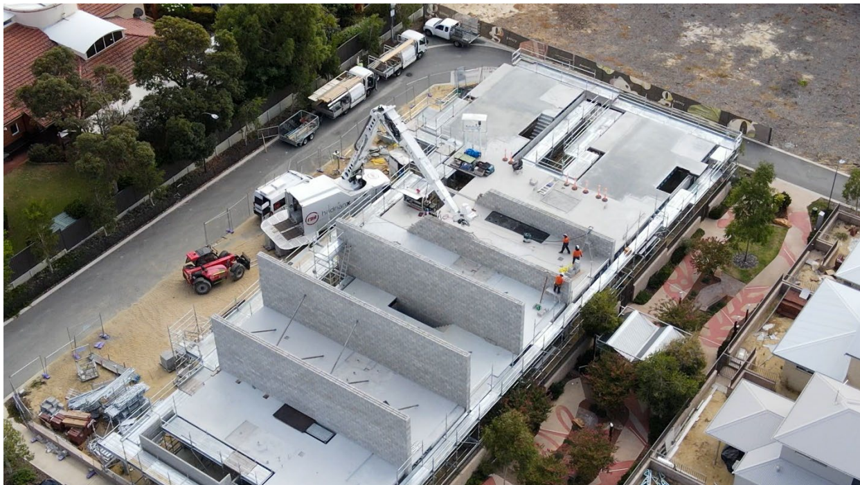
H02 completing the second storey common-party walls of the final stage at Willagee
