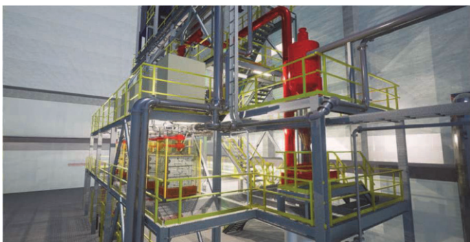
Figure 6: In-house designed packed bed calciners
