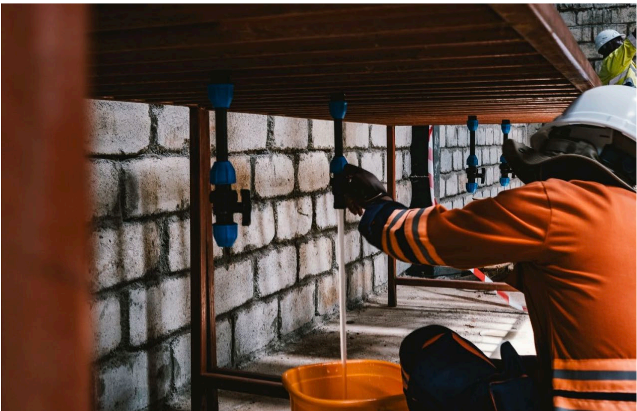
Figure 6: Water commissioning of desorption columns.
