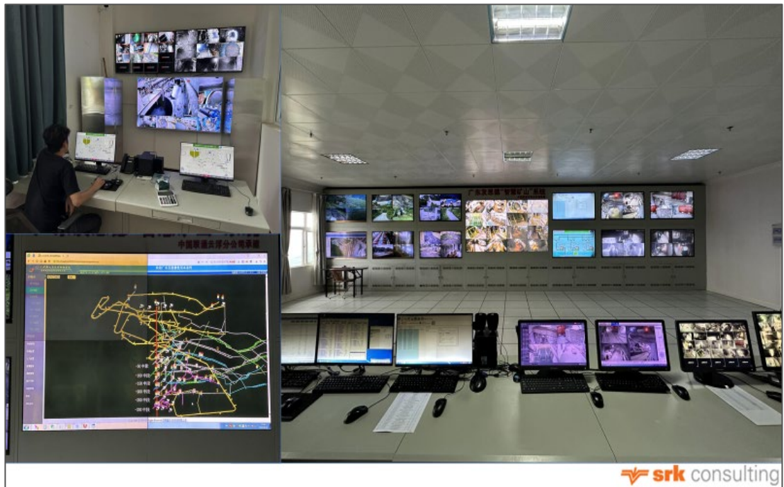
Figure 6-13: GC Mine Central Control System
