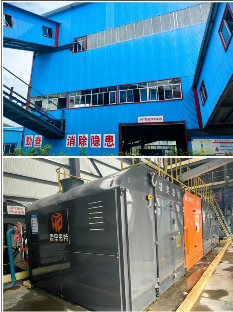
Figure 6-3: The Intelligent Preselection System plant
