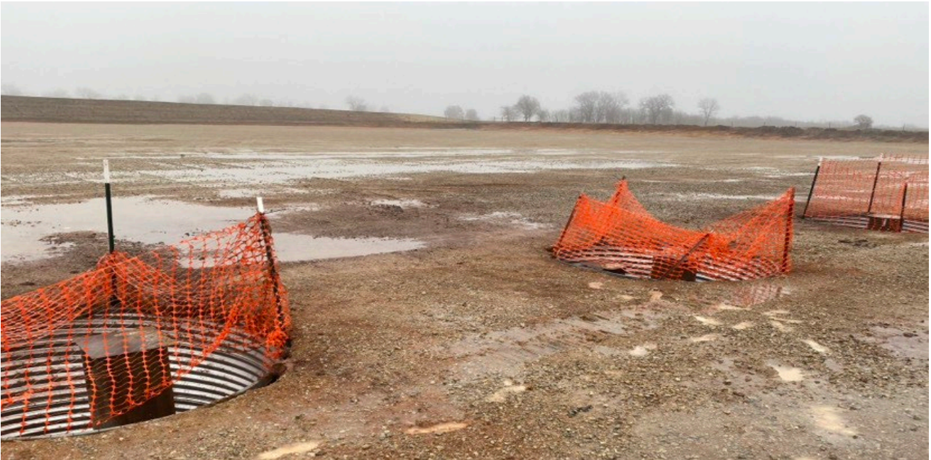
Figure 2: 80-foot conductor holes set for each of the Fleury, Maroons, and Iginla Wells on the Sanford Pad in preparation for drilling operations.
