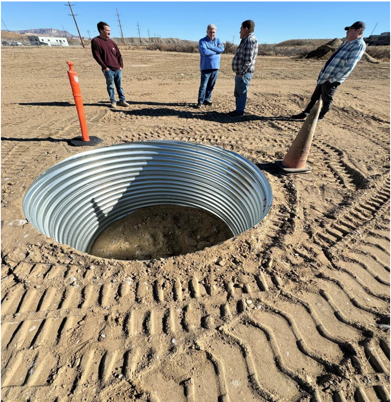
Figure 1: Photo showing the “cellar” for the planned well with the visitor centre in the background on Anson’s privately owned Green River property with a Green River Councilor and a local contractor.
