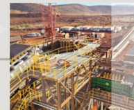
LOAD OUT INFRASTRUCTURE
