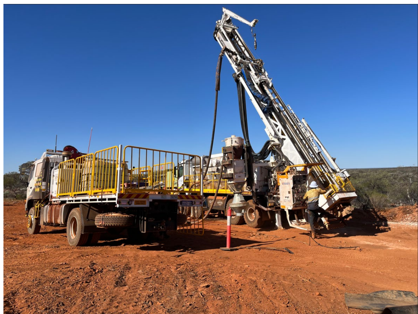
Figure 1. Orelia Target 1 – Drill Rig set up on the first hole at Orelia.
