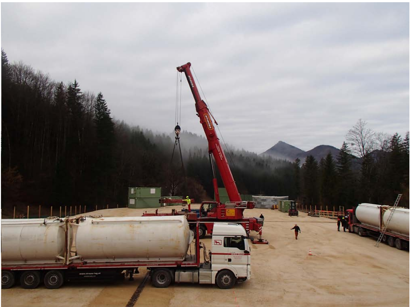
Figure 1: Commencement of rig up of the RED E200 drilling rig at the Welchau-1 drilling location
