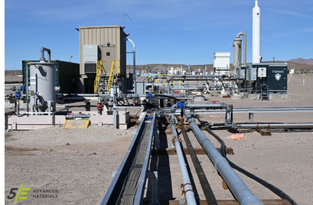
Figure 2: Photo of wellfield DCS Feb 2024
