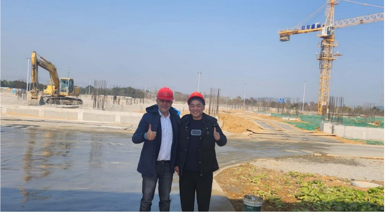
Photo: Vmoto's Managing Director, Mr Charles Chen and Chief Marketing Officer, Mr Graziano Milone, at the building site of Vmoto's Stage 2 Manufacturing Facilities.
