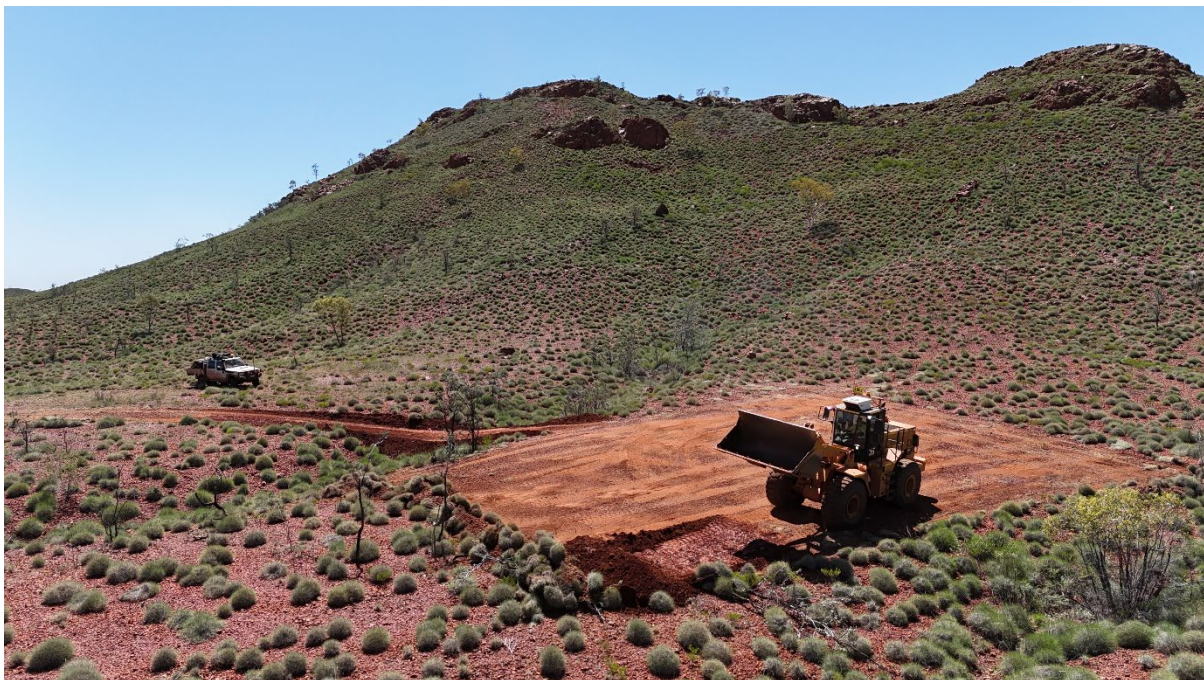
Figure 1: Drill access and pads have been completed for upcoming drilling scheduled to commence in the coming weeks.
