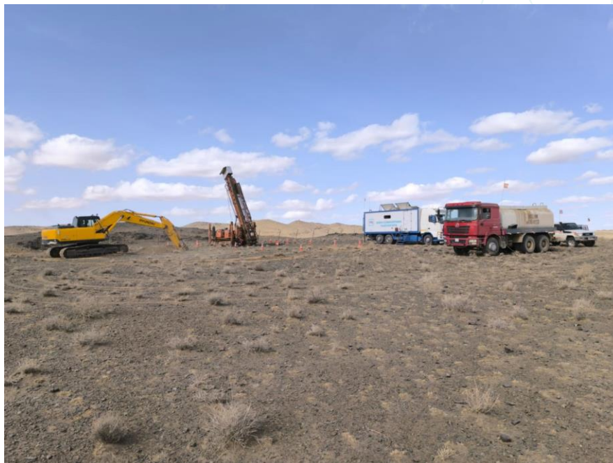
Figure 2: Drill rig and lab ready for the resumption of Drilling at the BNG Project
