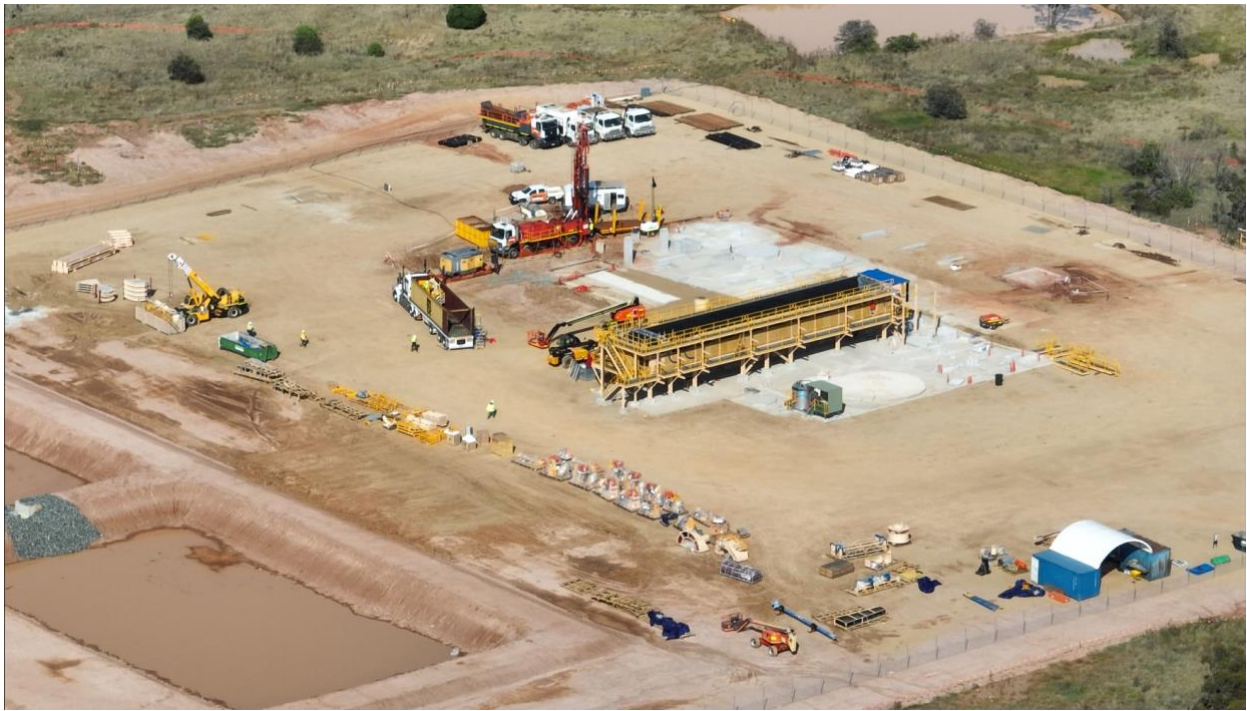
Paste plant concrete and belt filter
