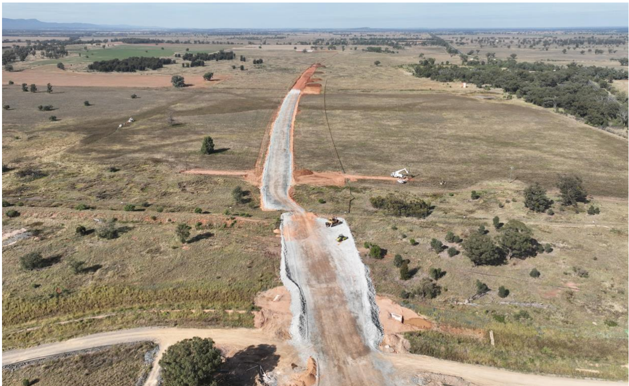
Internal light vehicle and pipeline corridor construction between Caloma Two and Roswell
