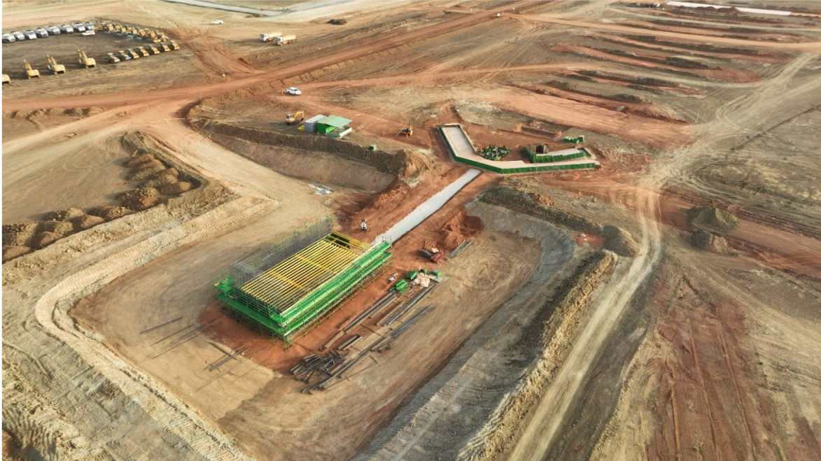
Kiaka Primary Crusher Area
