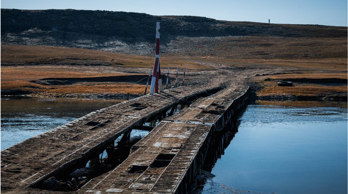
Figure 7. Example of current underdeveloped infrastructure in region impacting on safety and reliability of transportation.
