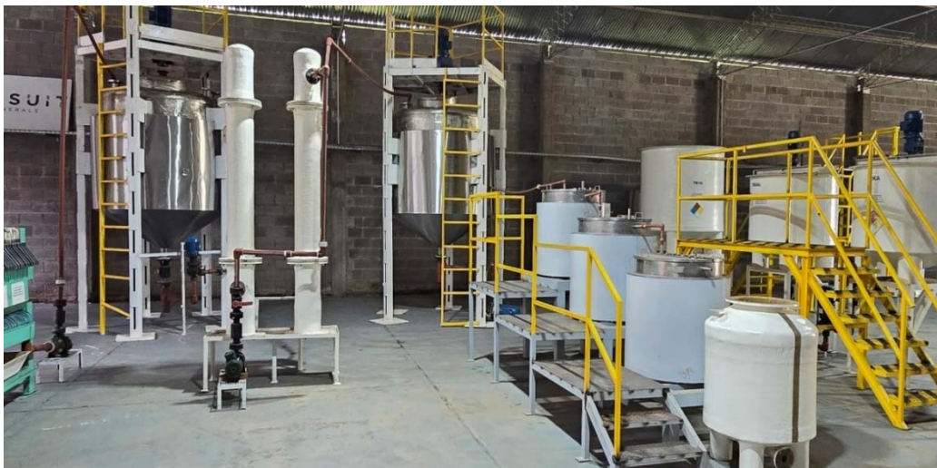
Figure 6: 250tpa Lithium Carbonate Plant at Pursuit's purpose facility in Salta, Argentina
