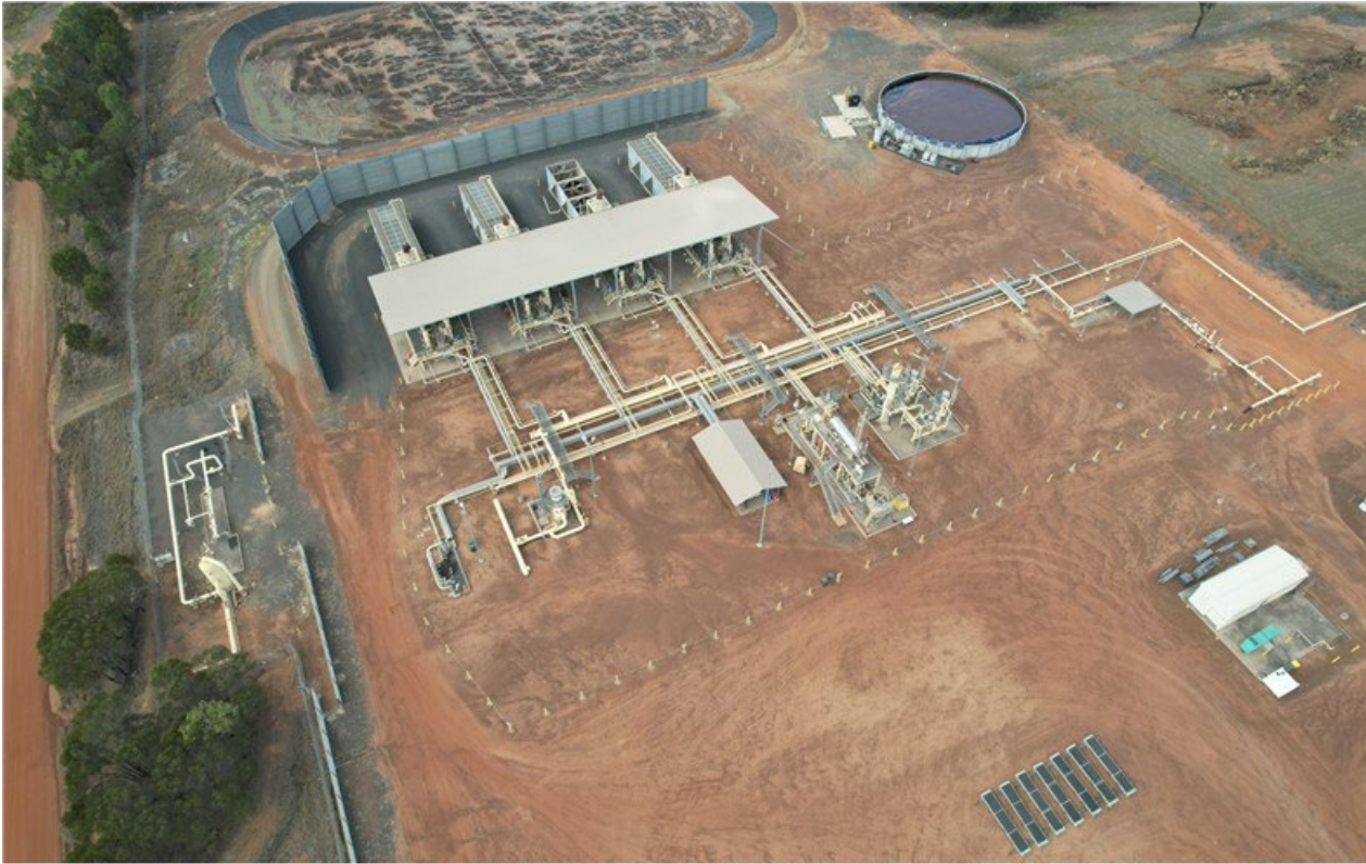
Moranbah Gas Processing Facility
