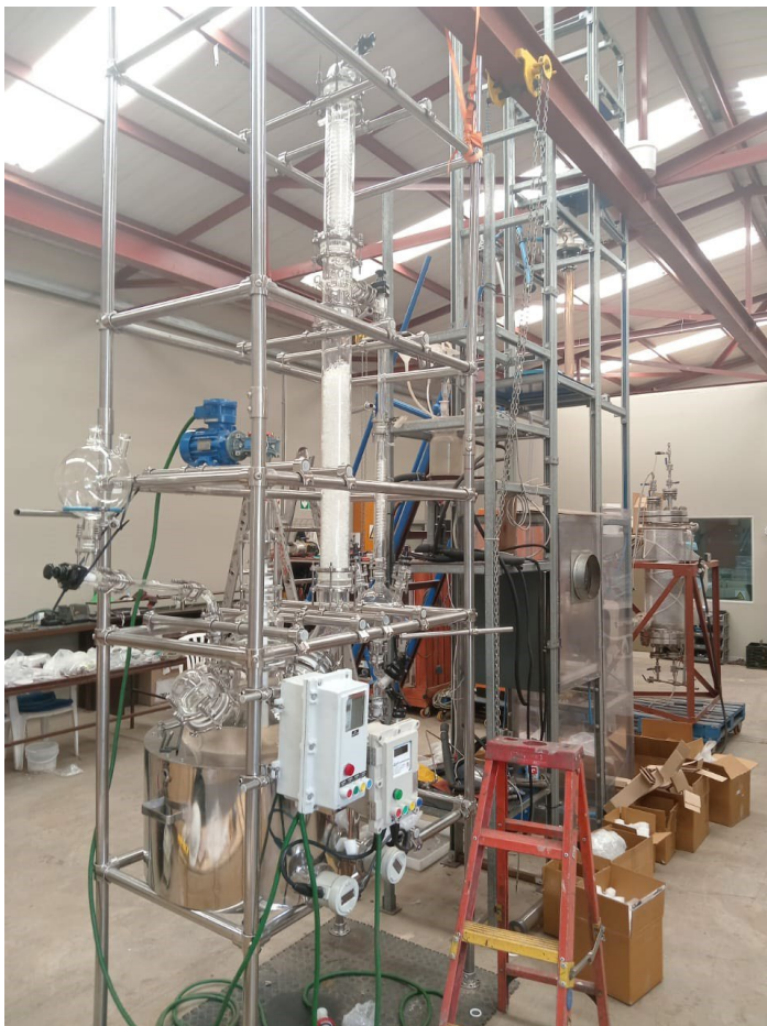
Figure 1: Distillation column for Globe's Pilot Plant under construction at Resonant Group's facility in Johannesburg, South Africa.
