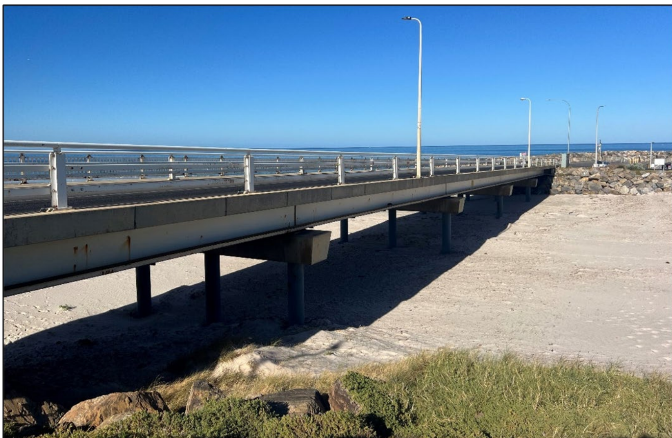
Figure 2: Trial infrastructure at West Beach Bridge, Adelaide, SA
