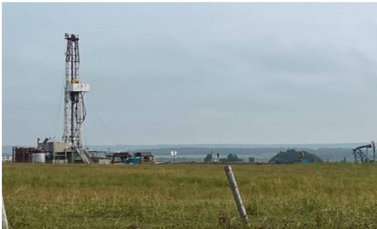
Figure 1. Caroline Liquids Rich Gas Well Site
