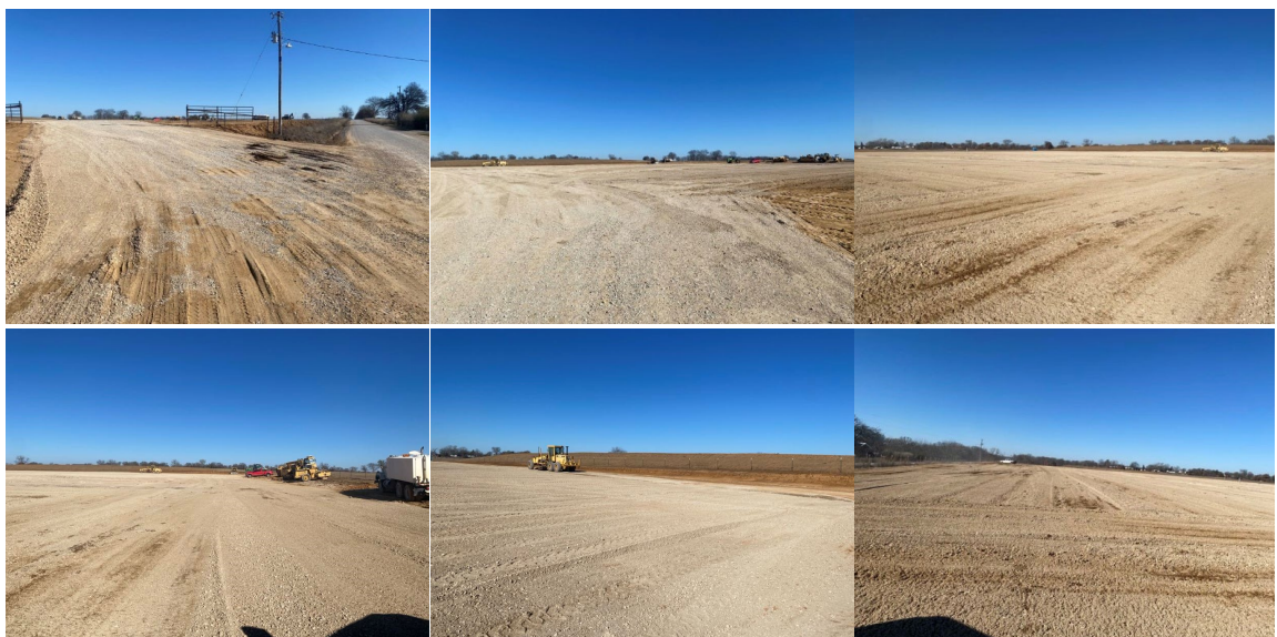
Figure 5: Construction of the Sanford Pad from which the Iginla, Fleury and Maroons Well will be drilled.
