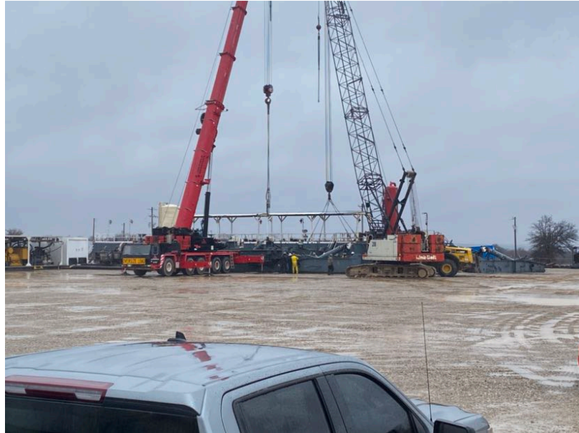
Figure 6: Kenai Rig 19 setting up on the Sanford Pad in preparation for spudding of the Iginla well, the first of four in the multi-well FMDP.
