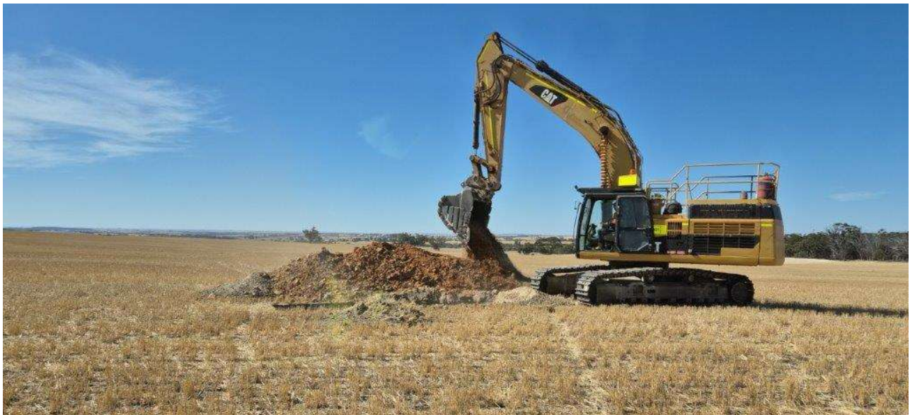
Figure 3 – Excavator digging a geotechnical test pit beneath the planned Tailing Storage Facility (TSF).
