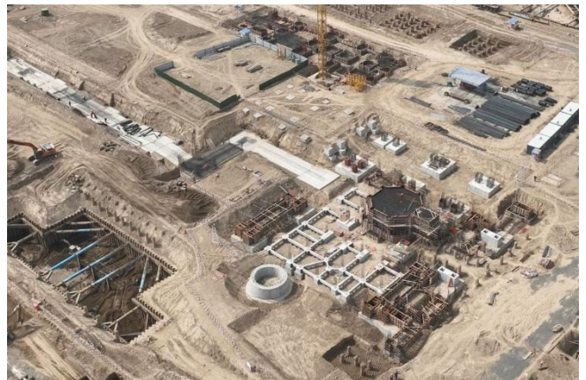
Figure 1 Latest photo showing the smelt reduction vessel (SRV) and forehearth foundations of the latest Hismelt plant being constructed in Hebei province, PRC.
