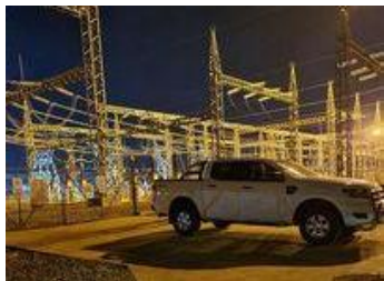
Eskom Substation 12km away
